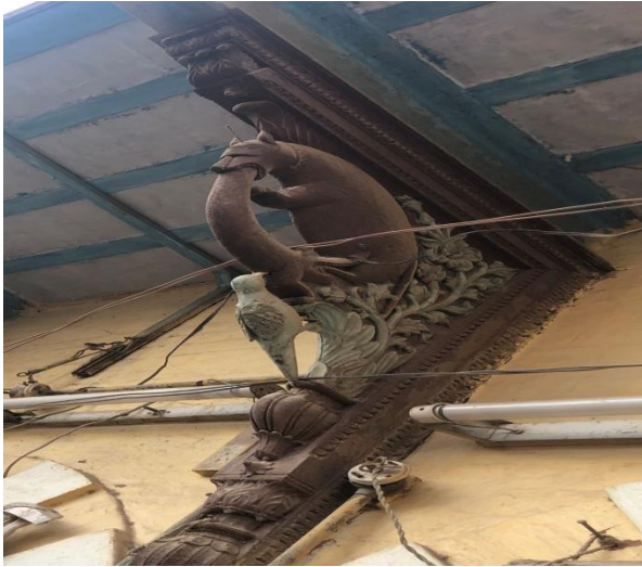
Figure9: shows the wooden craft work under projected I beam (Guarder). (at Awan Muhalla).
