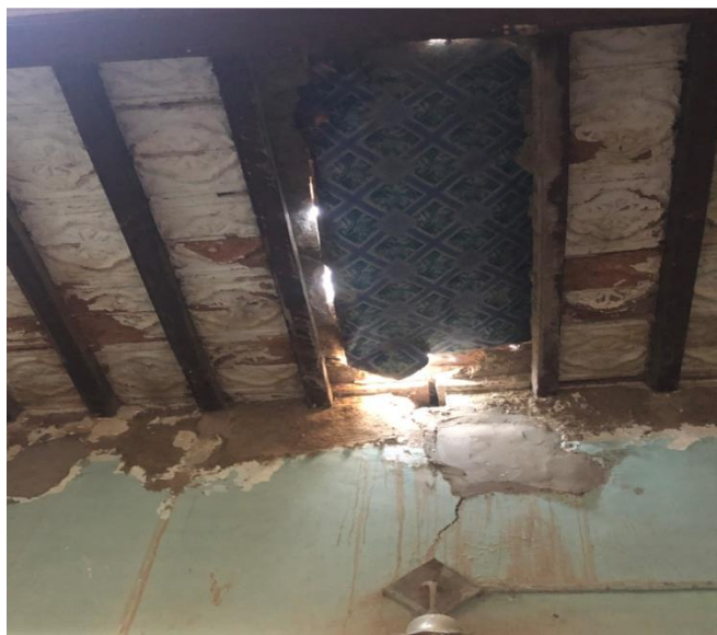
Figure5: shows the roof built by rafter and burn bricks. (a house built in 1930 at Awan Muhala)
