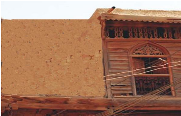
Figure 3: shows the wooden frame reinforcement in of same house covered with plaster.
